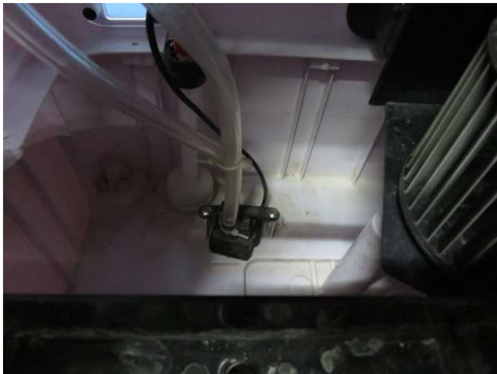
Water pump view
